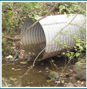
Fish are unable to swim through culverts that are too long or perched above the water, like this one on Hawthorne Drive Creek.
